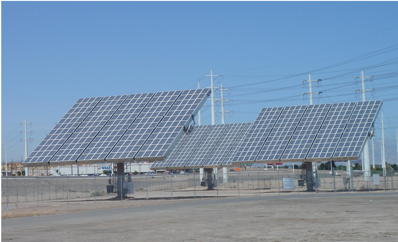
Figure 2. A 75 kW installation for Nevada Power in Las Vegas, Nevada. The systems were installed May 2006.
